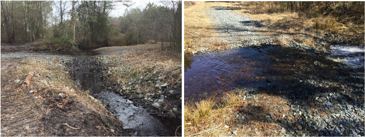
Figures 5a and 5b. Rock weir spillways installed within a surface drain to restore wetland hydrology. In these cases, the spillways also function as fords for occasional vehicle crossing.
