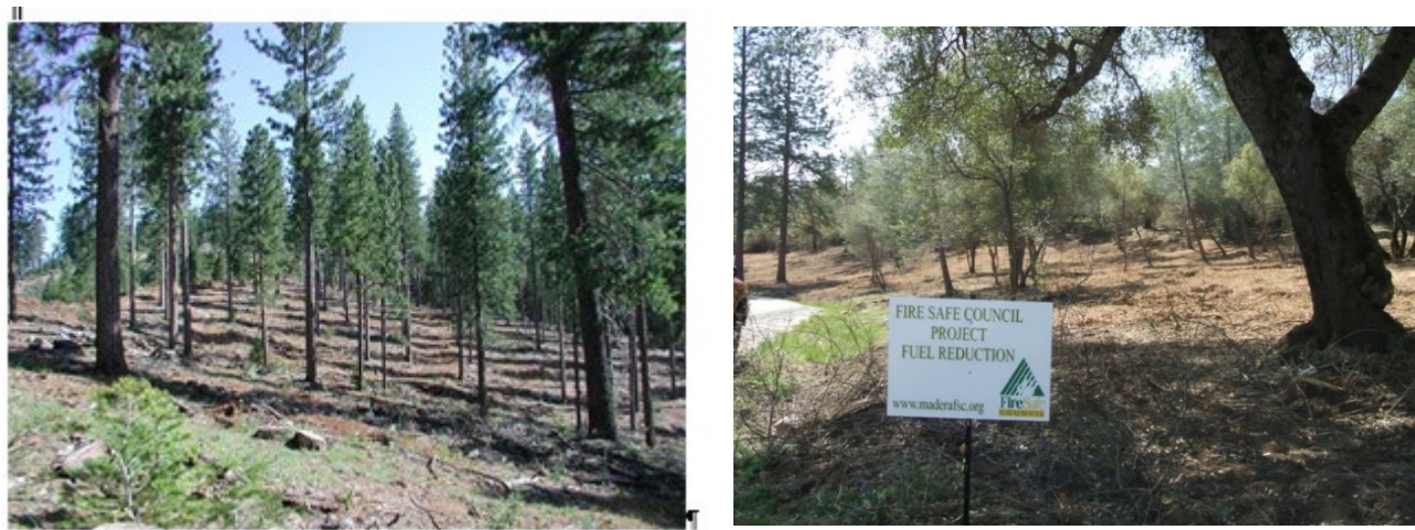
Figure 1. A fuel break on forest land involves the reduction of flammable fuels, eliminating ladder fuels, and increasing the spacing of residual trees in order to minimize the risk of crown fires.
