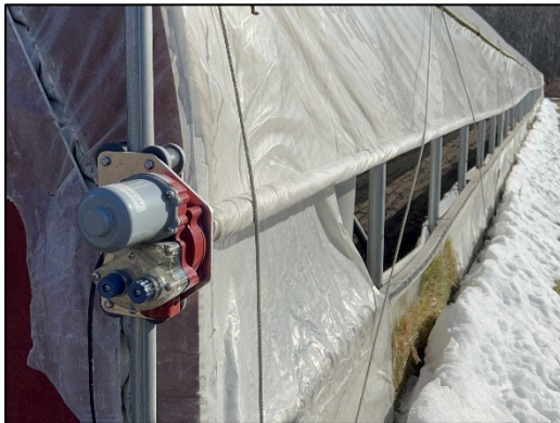
Motor and roll-up sidewall in operation to provide ventilation on a warm winter day.
