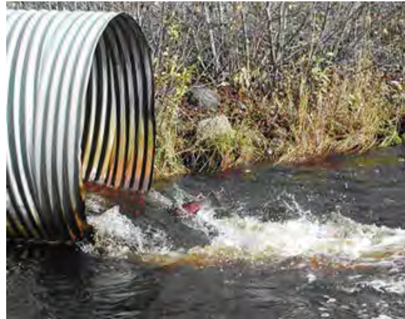
Figure 45: Culvert outlet drop, with Coho.
