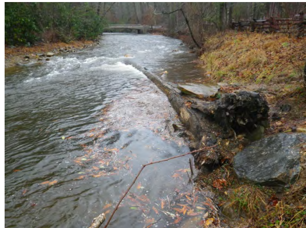
Figure 54: Log J-hook vane providing bank stabilization and pool scour 4 years after construction (Pisgah National Forest, North Carolina; photo credit: Brady Dodd).
