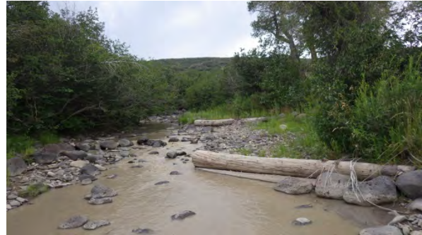
Figure 53: Log vanes at low flow providing bank stabilization and channel narrowing 2 years after construction (Milk Creek, Colorado).
