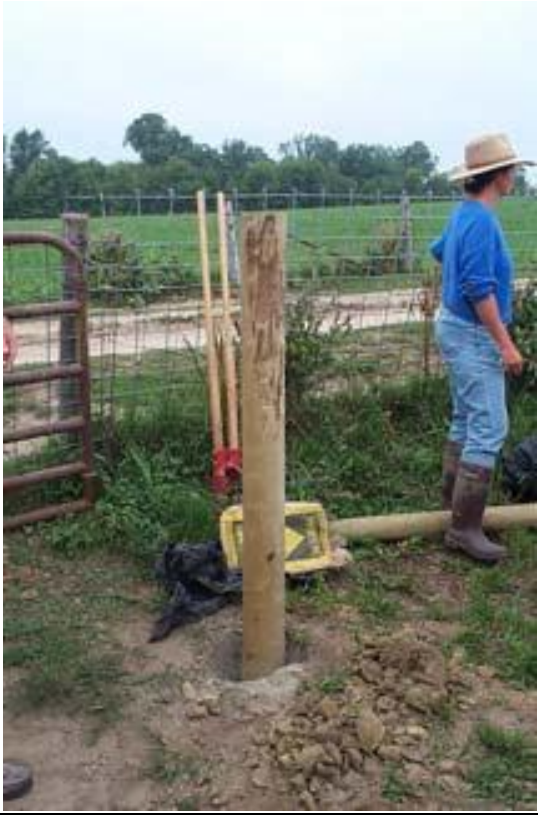
Dig in post hole and tamp earth in lifts or drive post
