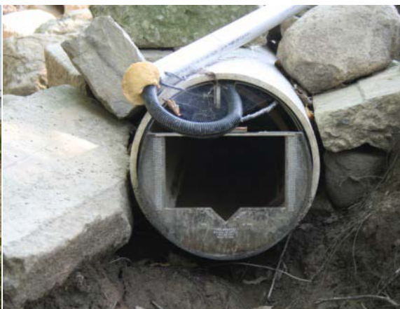
Figure 2: Subsurface tile drainage pipe with Thel-Mar compound weir.
