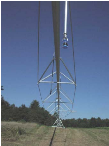
Sprinkler heads on center pivot.
