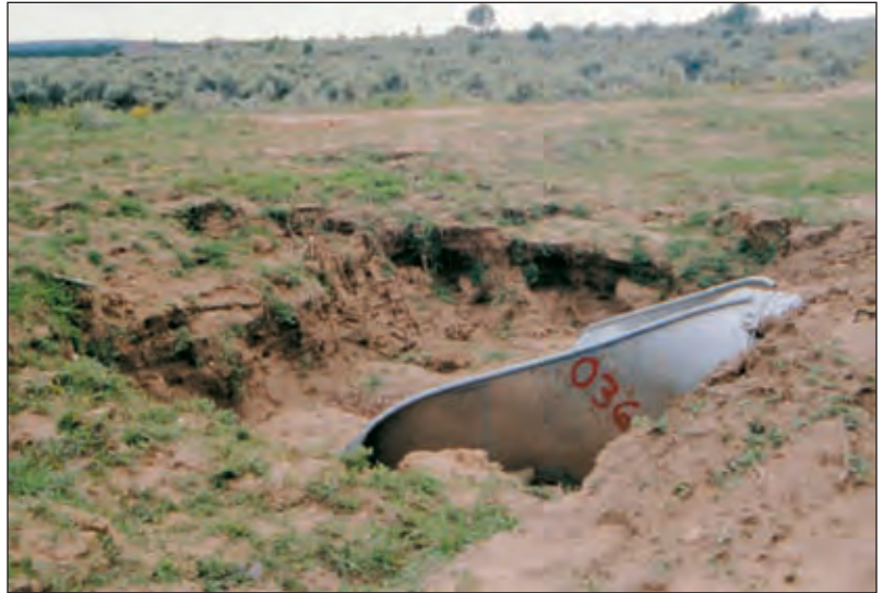
Photo VIII-2: Headcutting caused by improper culvert installation.
