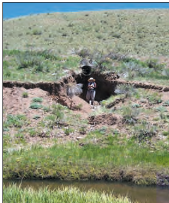
Photo IV-3: This cross drain culvert was installed at a point where the soil could not absorb concentrated runoff and should be relocated to a more favorable site that can filter and absorb road runoff.
