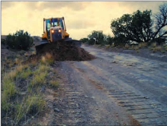
Photo V-4: Removing the unwanted berm will allow surface runoff to spill this outsloped roadway.
