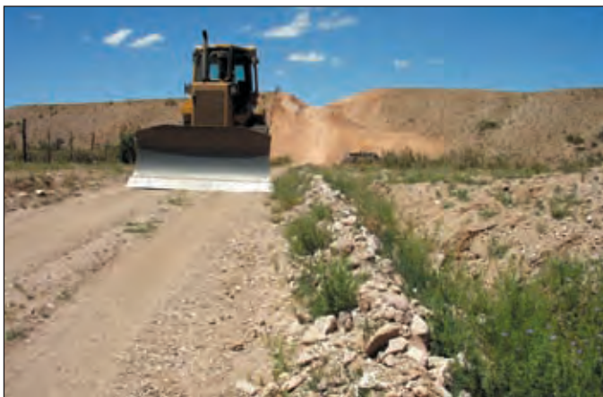
Photo V-1: A crowned road. The berm on the right must be removed to assure drainage to the road ditch.
