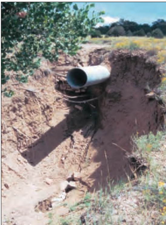
Photo V-12: This 18-inch diameter corrugated steel pipe had adequate cross slope, but no energy dissipater.
