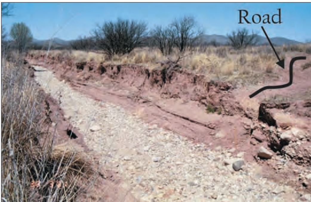
Photo III-2: Straightening of the channel at an unpaved ford caused this channel bed to down cut.
