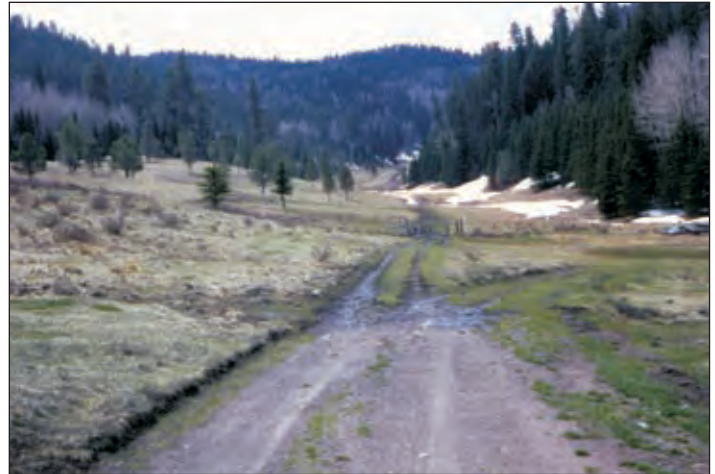
Photo II-1: Valley-bottom roads can be difficult to drain.
