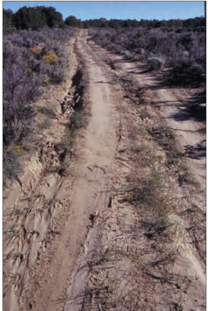
Photo VII-1: Flow patterns show where drainage structures have failed.
