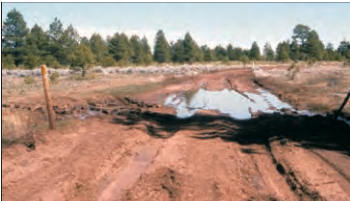
Photo VII-2: Puddle formation due to too little slope in the dip drain.
