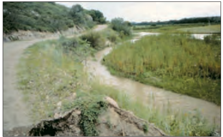
Photo VIII-4: Road encroachment on streambank.
