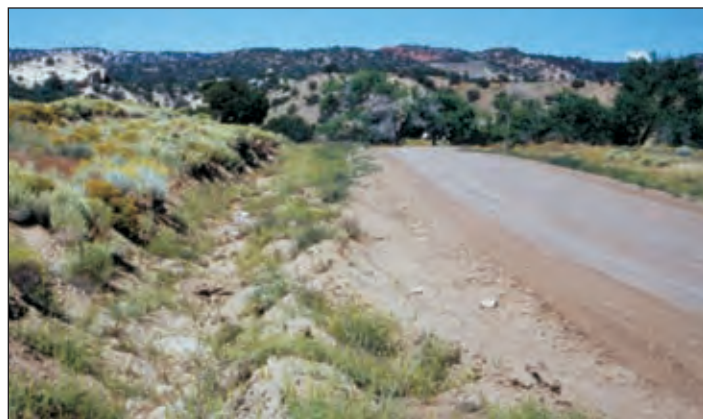
Photo III-1: This berm keeps water from the road surface from spilling into the road ditch.
