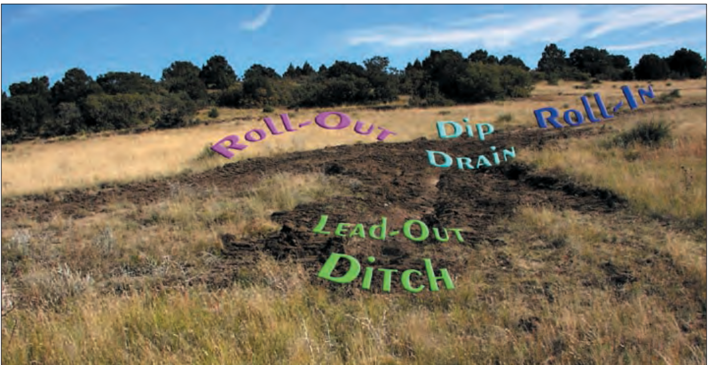
Figure V-3: Key features of a rolling dip are the dip drain, lead-out ditch and roll-out.
