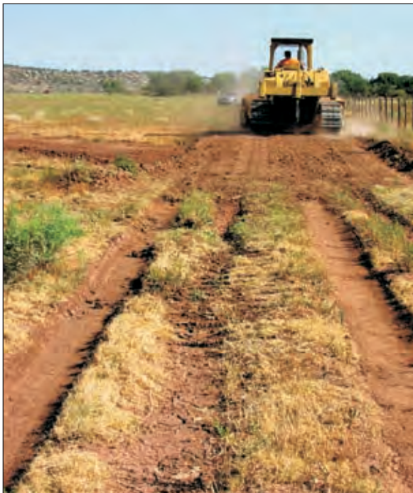
Photo V-10: Tractor constructing reverse slope ramp beyond lead-out ditch using the stockpiled fill (photo V-9).
