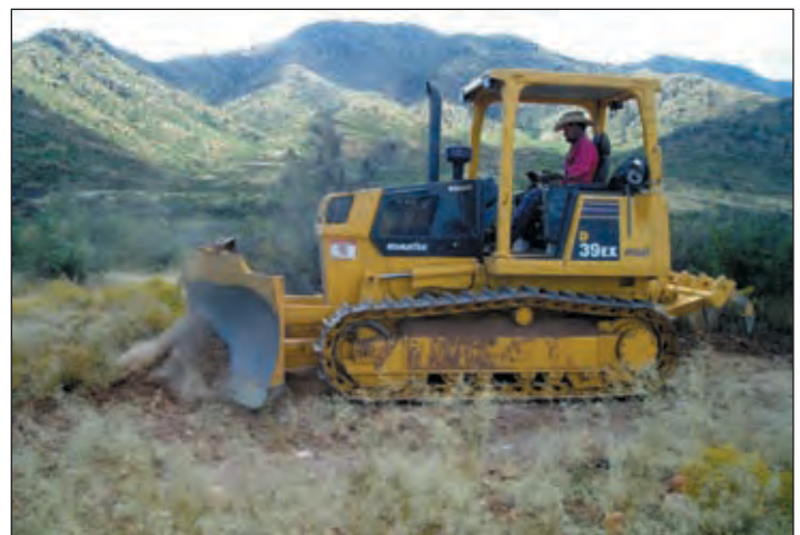
Photo IX-1: A medium sized bulldozer is ideal for building cross drains and for most maintenance situations.
