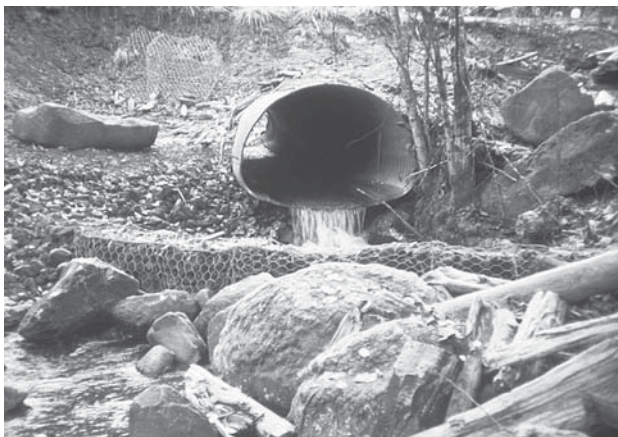
Figure 6-12. A complete fill washout because of a plugged culvert inlet.
