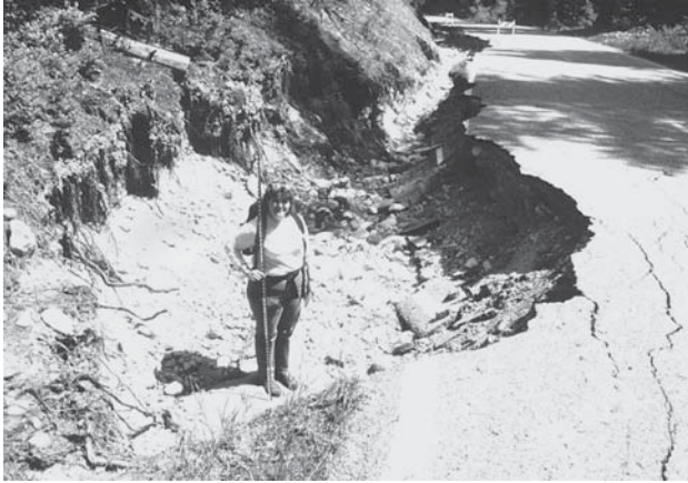
Figure 6-11. Significant ditch erosion.
