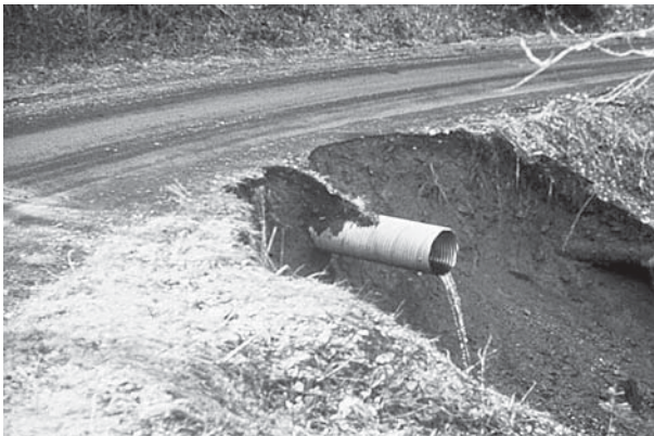
Figure 2-8. Erosion caused by a culvert in need of a downspout.
